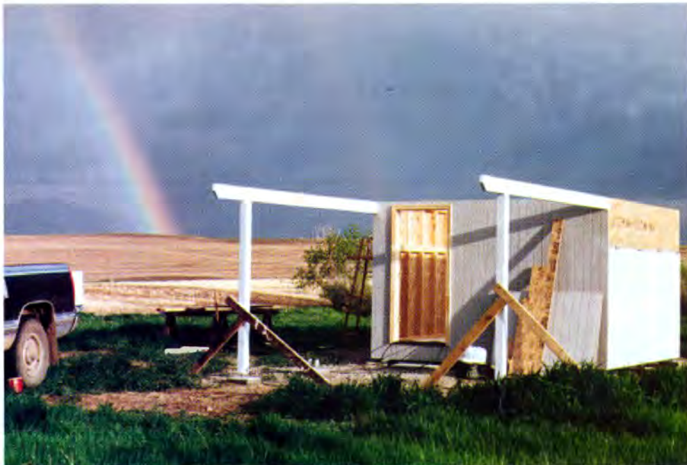
AT THE END OF PHASE 2 , the floor, walls, fold-down wall sections, and roll-off roof rails are in place. A good coat of exterior-grade primer will shield the structure from the elements until we can install the roof in part 3 of this series.
