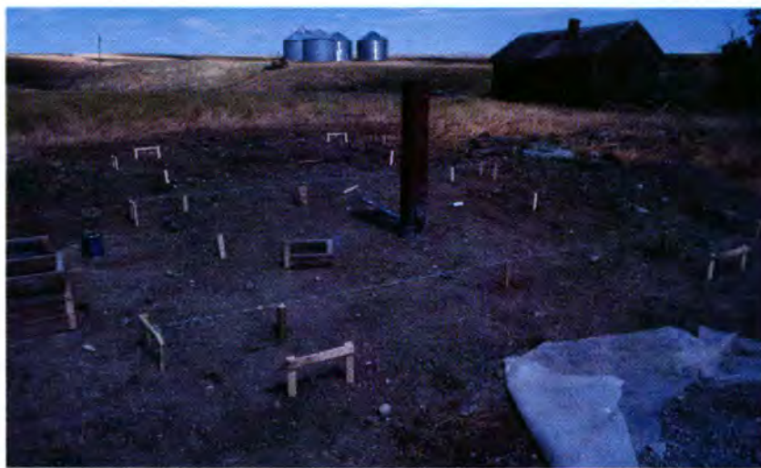
TWELVE FOOTINGS FORM THE FOUNDATION. Using the dimensions from the plan at top, stakes were first driven at the corners of the structure (above). To locate the holes for the footings, batterboards and strings were placed outside the stakes.
