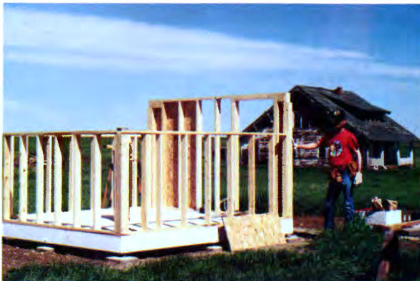
RAISING THE WALLS is easy once the prefabricated sections are delivered to the site (top). The north wall is erected first and held in place with a temporary support. The west and east walls are fastened to the north wall (middle). Finally, the south wall is screwed in place (bottom).
