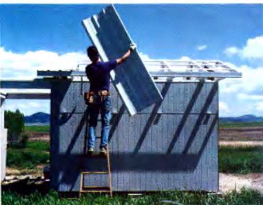
RAISING THE ROOF starts with pre-assembled king-post trusses that are screwed to the joists in the rolling frame and ends with corrugated metal roofing that attaches to three 1x4 stringers (photos from top to bottom).
