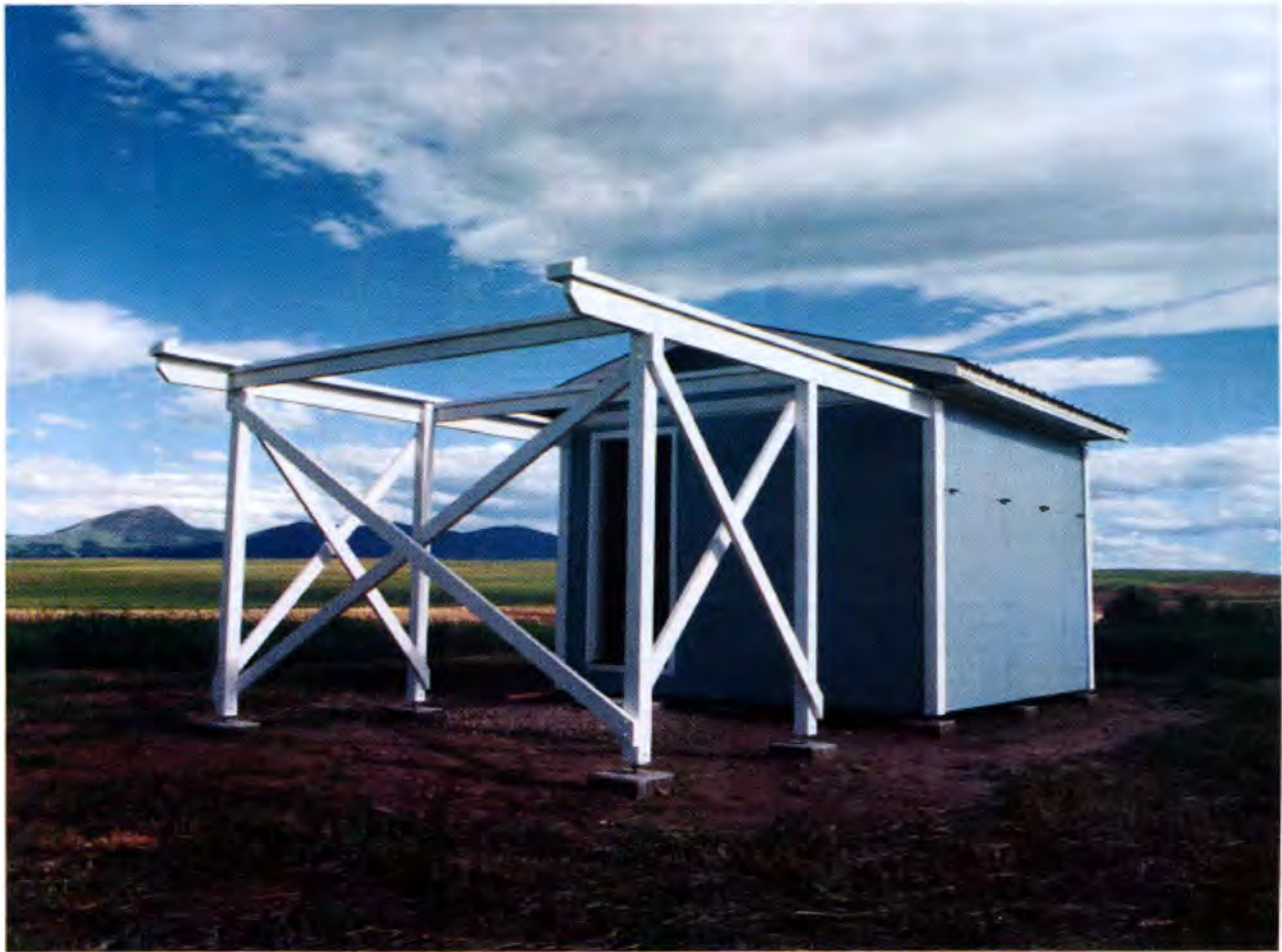
THE FINISHED OWL OBSERVATORY has siding installed in the gable roof ends and along the roof eaves, corner boards made from 2x4s, the door replaced, door trim, and a coat of exterior paint.
