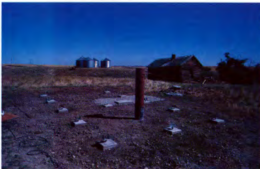
AT THE END OF THE FIRST PHASE OF CONSTRUCTION , the concrete footings and pier have been cast and the observatory site has been raked level in preparation for the construction of the floor and walls.
